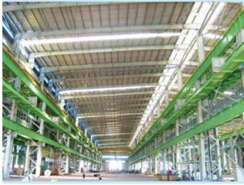
Multi-Level Crane Beam
