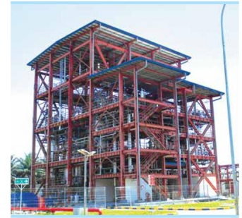
Hydrogenation Plant (Indonesia)
