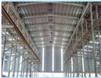
AHT Steel Mill - 1,000 MT
