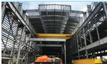
BSRM Steel Mill (Bangladesh)
