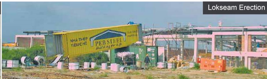
Lokseam Processing @ Site
